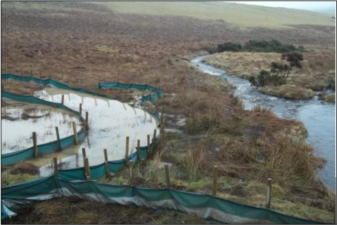
Plate 5.2: Photograph of Silt Fencing
