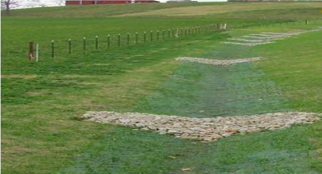
Plate 5.3: Photograph of Check Dams
